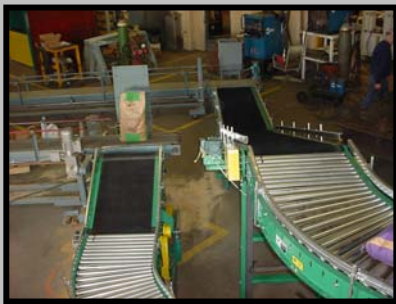
Bag Conveyors at Fill Lines
